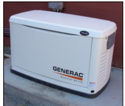
The new generator with automatic transfer which runs the whole building when the power goes out!
